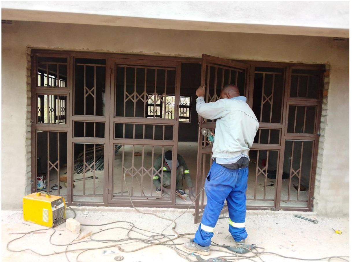
The outstanding 4m door was made successfully and fixed to the structure
